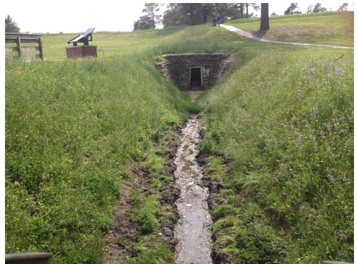
Entrance to the 511 foot Federal tunnel. Photo taken on May 3, 2013 by Battle Cry editor.
